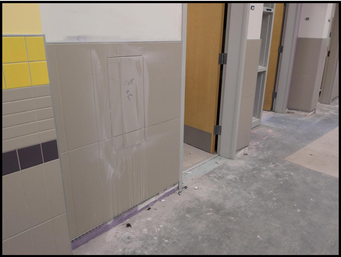
Cut in fire extinguisher cabinet at C-2 corridor ceramic tile – 05/26/26
